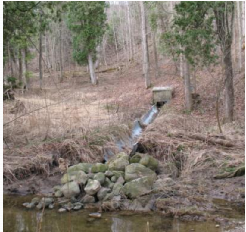
STP Outfall at River
